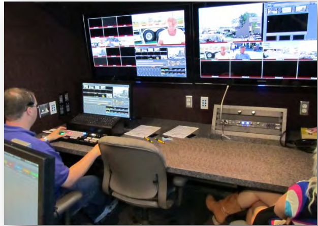
Video Control Room front desk 1
